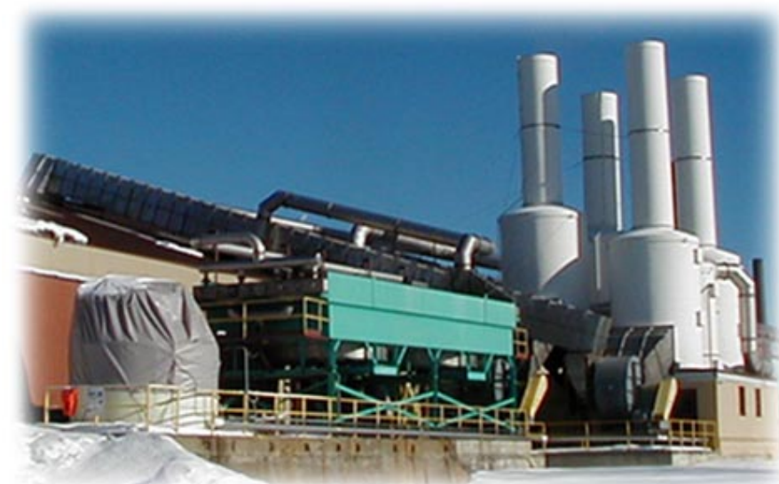
Baker Commodities is proud of their modern odor control system at their Massachusetts plant, which was totally rebuilt after a devastating fire in 1996.
